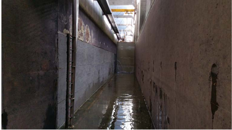
Cleaned Side Dewatering Screen
