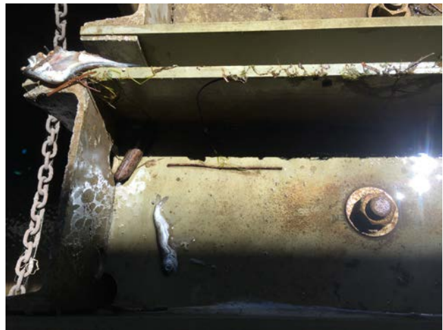
Emergency Bypass Bulkhead Fish Mortalities
